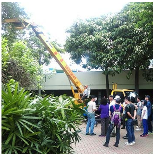
LCSD staff watched a demonstration on the use of hydraulic platforms for tree work.
